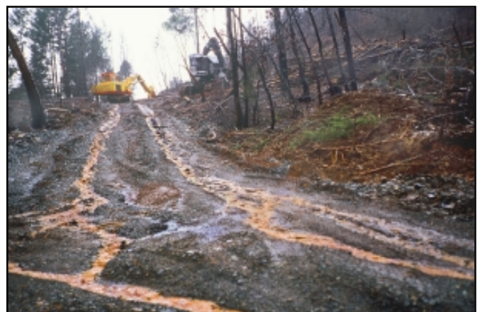
Private land salvage logging in the Biscuit fire area near the Wild and Scenic Illinois River shows how the fragile soils easily erode. Photo by Rolf Skar.
